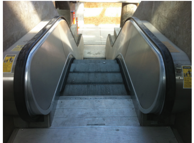
LAX's New elevators and escalators use energy saving, sustainable technology.
