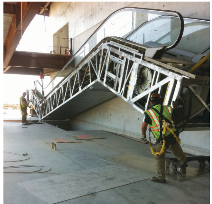
New elevators and escalators will speed travelers to their destinations in a safe and energy efficient manner.
