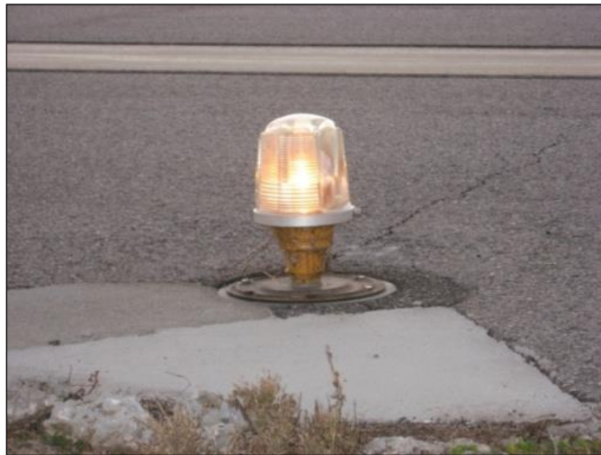
Elevated Runway Edge Light Fixture
