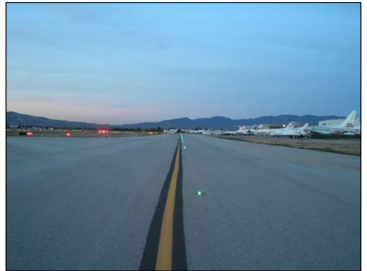
Taxiway Centerline Lights
